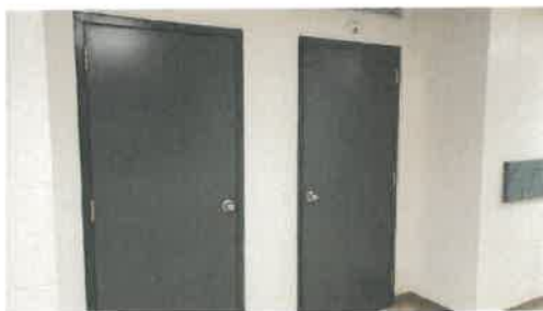
Most classrooms have solid doors with no sidelites. This creates a closed off classroom from the corridor.
