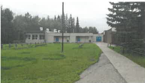
The existing 1977 modular classrooms are in poor condition and require replacement.
