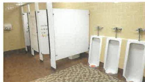
Barrier-free access needs to be improved for all washrooms in terms of stall size, counter heights and clearances, and urinals.
