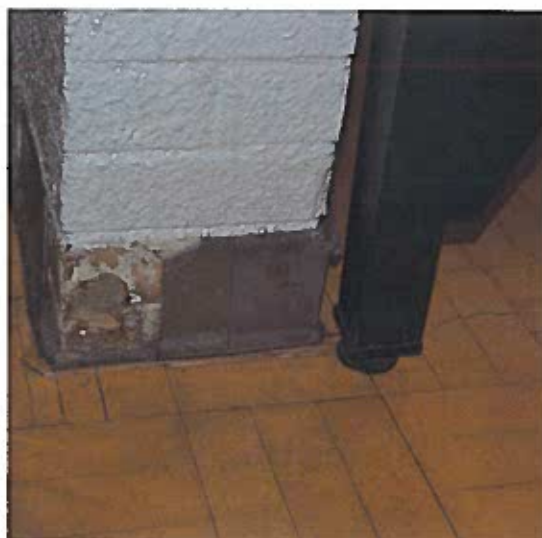
Left - Washroom Right - Damaged wall base
