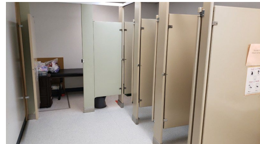
Barrier-free access needs to be improved for all washrooms in terms of stall size, counter heights and clearances, and urinals.
