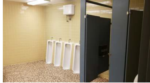
Barrier-free access needs to be improved for all washrooms in terms of stall size, counter heights and clearances, and urinals.
