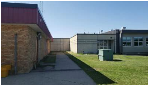
It has been identified that there are a number of areas around the school that have issues with drainage at the walkways and ice forming in the spring.
