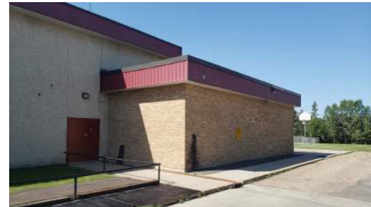
The staff parking area and North access lane flood frequently.
