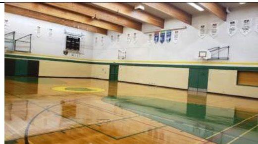
Acoustic baffles are required in the gym to reduce reverberation.
