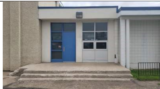
Entrances require upgrades to meet accessibility and building code requirements.
