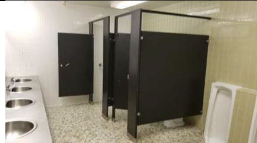
Barrier-free access needs to be improved for all washrooms in terms of stall size, counter heights and clearances, and urinals.
