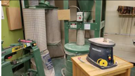
The dust collector in the industrial arts area may not be adequate and should be reviewed in relation to current code requirements.
