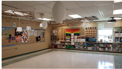
A large number of classrooms have a lack of natural light, low ceilings, hanging plug-in lamps with extension cords in the ceiling spaces, and an abundance of fluorescent lighting to compensate for the lack of natural light which is a challenge for students and staff who struggle with fluorescent lighting.
