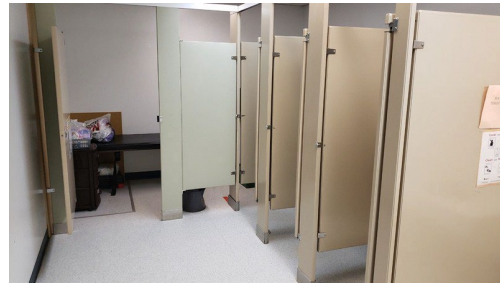
Barrier-free access needs to be improved for all washrooms in terms of stall size, counter heights and clearances, and urinals.
